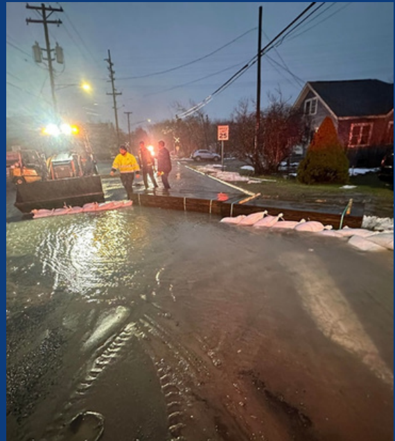
Neighbors helping neighbors! When the City of Northville experienced a devastating water main break, City of Plymouth DMS crews brought over sandbags to help direct the water away from homes.
